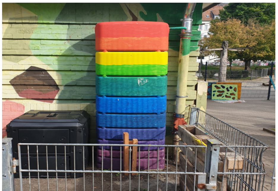
© iResilience: installed water filling station Dortmund Harbour neighbourhood
